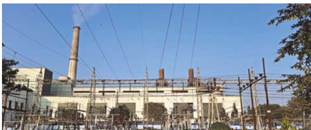
Bandel Thermal Power Station
